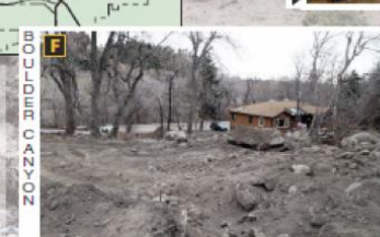
This debris fan along Boulder Canyon Road (Highway 139) impacted the rear of the home, causing half of the structure to move from its foundation. The fan also buried a portion of the parking lot. Location: 40°5'44.17"N, 105°17'50.02"W
